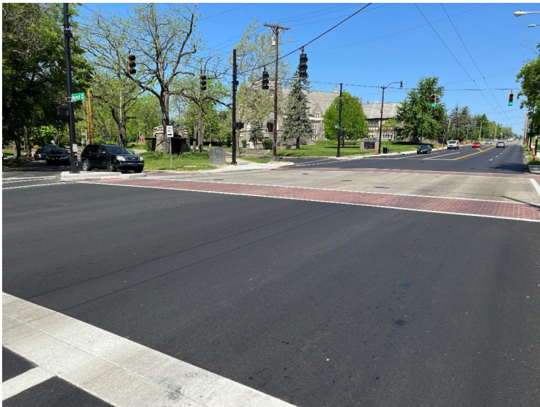
Photo: A portion of the recently completed first phase (Salem Avenue at Harvard Avenue intersection).
