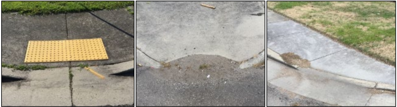
Examples of curb ramps that are less than the minimum 48" width required.
