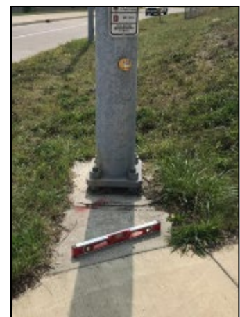
Example of pushbutton with non-compliant clear space adjacent.
