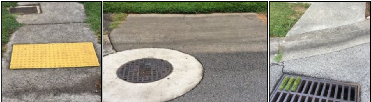
Examples of curb ramps with utility structures on the ramp or the clear space.
