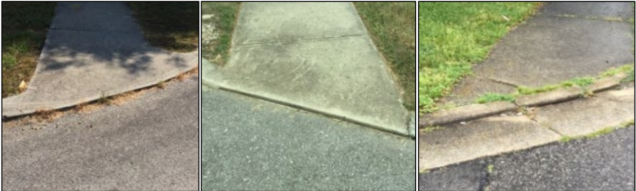
Examples of curb ramps with vertical discontinuities that exceed 1/2" at the curb, on the ramp, or the TS.
