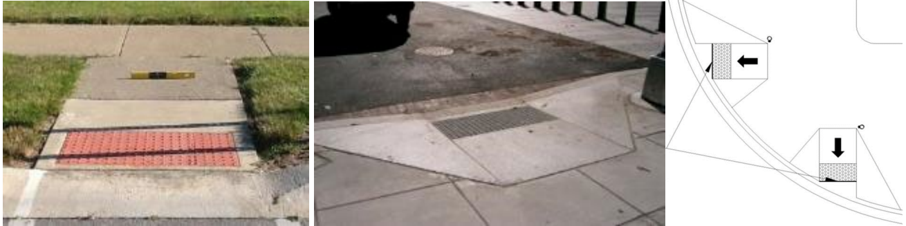
Example perpendicular curb ramps, with and without flares based on presence/absence of PCA.
