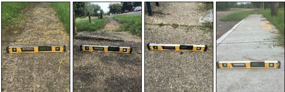
Examples of PAR with severe cross slopes and/or vertical elevation changes.
