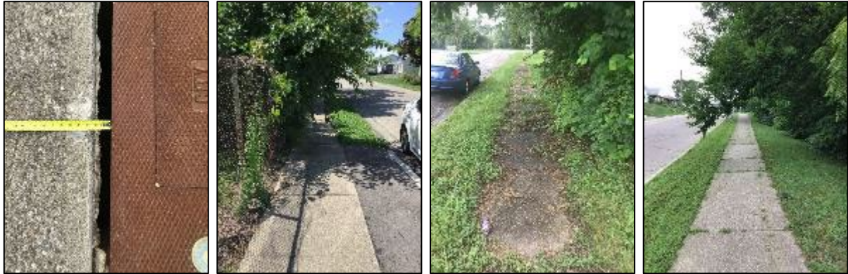
Examples of utility structure issues and vegetation obstructions/protrusions that can present issues for disabled users.
