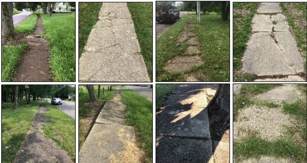
Examples of displacements, separations, and pavement in poor condition in need of maintenance.
