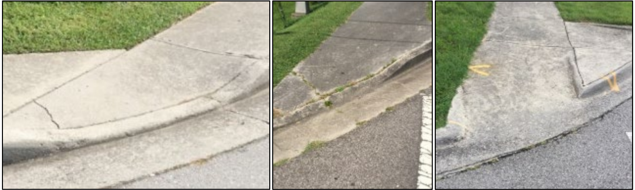
Example of curb ramps that have non-compliant flare slopes.
