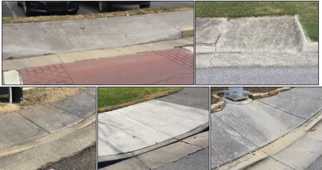
Example of curb ramps that lack a compliant turning space.
