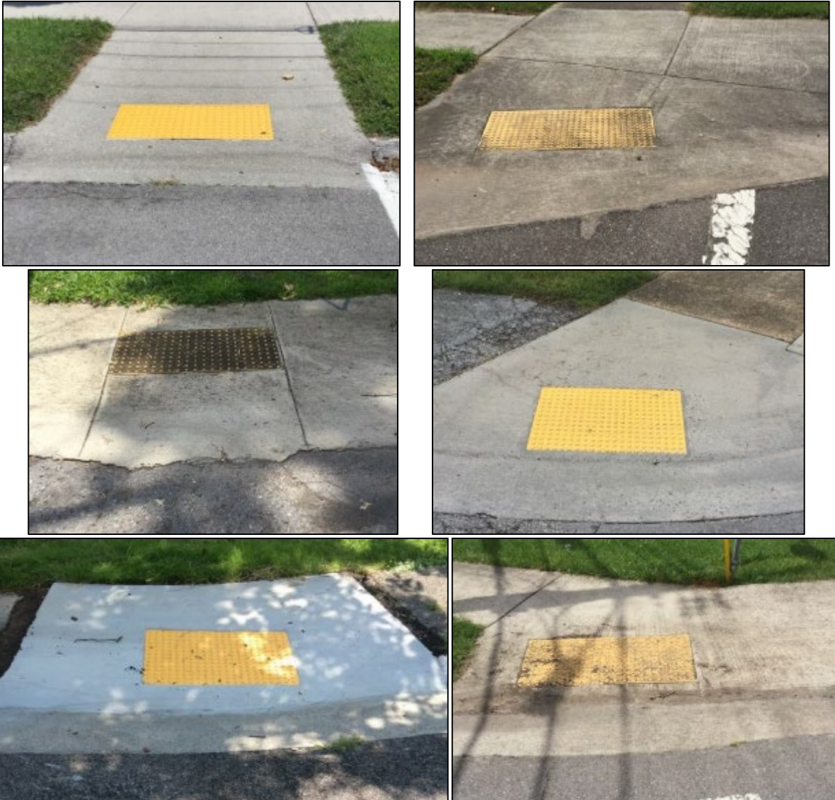
Example of curb ramps with detectable warnings that are not full width of the ramp.
