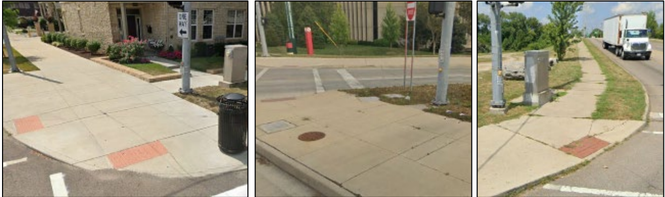
Example of pushbuttons that are outside the required 1.5-6.0 feet from the curb.
