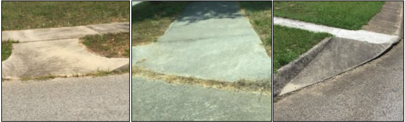
Curb ramps with excessive cross slopes. These ramps also typically have non-compliant landing cross slope.
