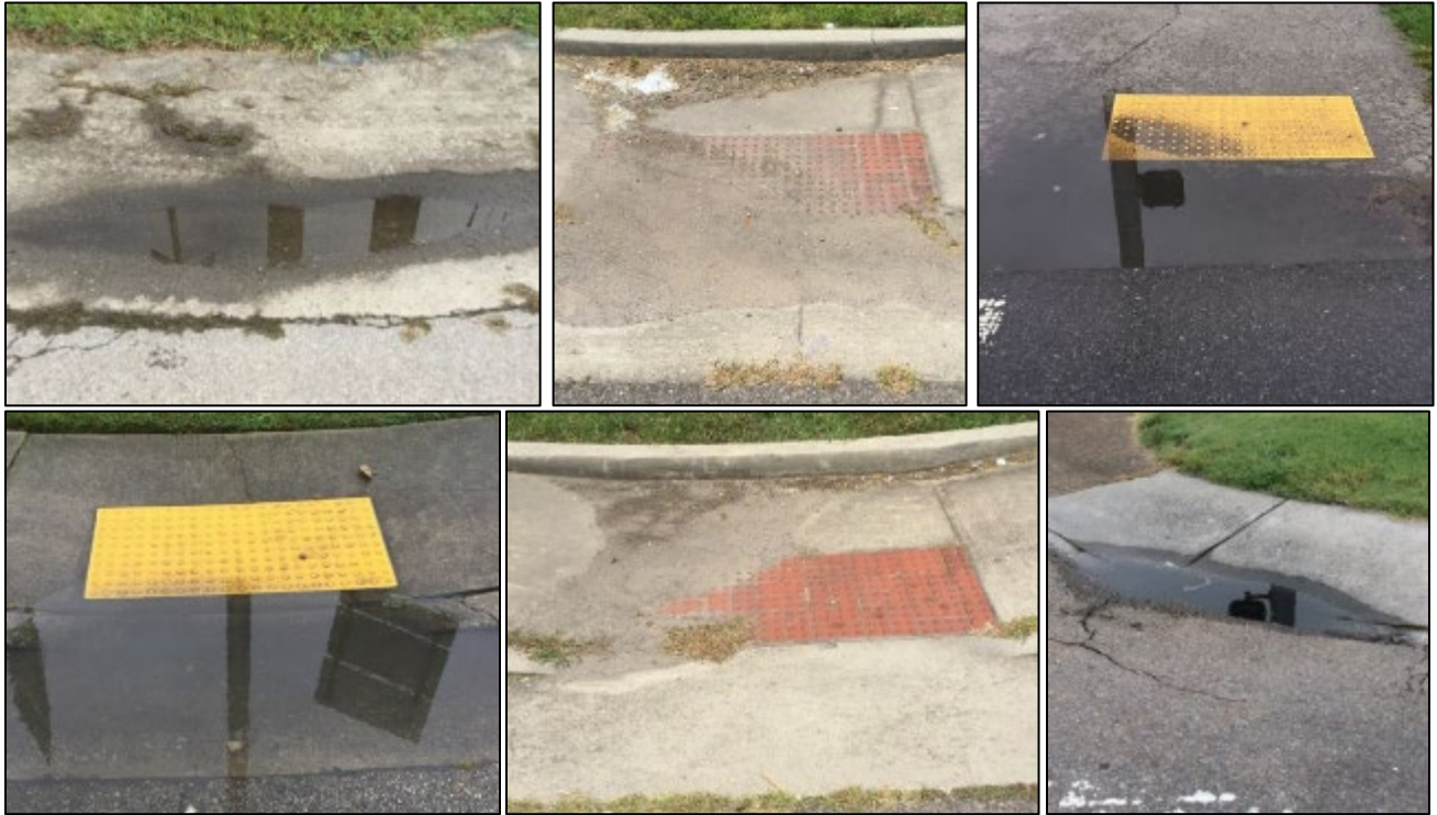
Examples of curb ramps with drainage issues and/or evidence of regular ponding, with sediment deposition.
