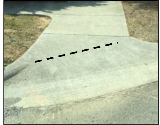
Example of curb ramp with a non-compliant grade break which is not perpendicular to the ramp path of travel direction.
